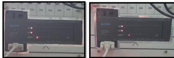
Figure 13: The Response of the PLC Unit to the Programming
