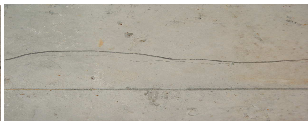
Fig. 6 Longitudinal cracks in web of box girder.
