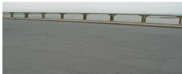
Fig. 12 Cracks of deck pavement
