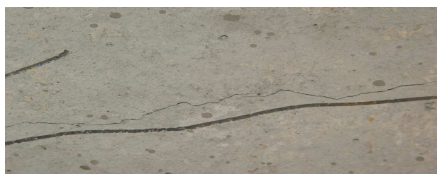
Fig. 5 Diagonal cracks in web of box girder
