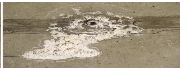
Fig. 4 Leakage of hole in the top of box girders
