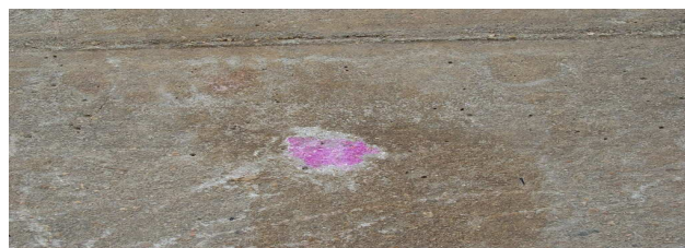
Fig. 17 Concrete carbonation of piers.
