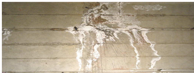
Fig. 3 White substance in the web of box girder
