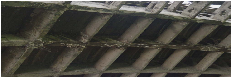
Figure 2: Cracks and water erosion of arch ribs
