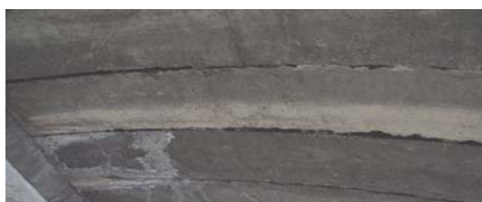
Figure 4: The damaged of arch plate
