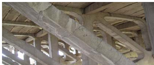
Figure 5: The cracks of the oblique truss bar
