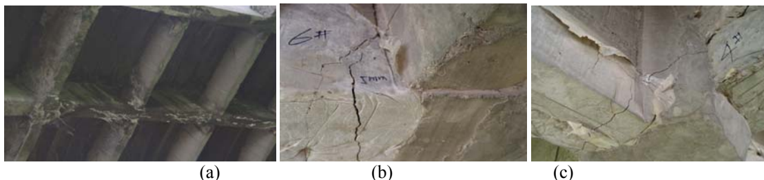
Figure 3: The damages of horizontal beam: (a) water seepage, (b) and (c) the cracks
