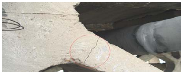
Figure 6: The oblique cracks of truss bar joint in the spans No. 5 and No.6.
