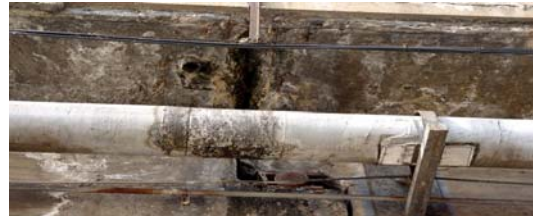
Figure 8: Damage of drainage system
