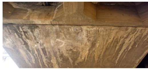
Figure 10: Damage of simply supported bridge
