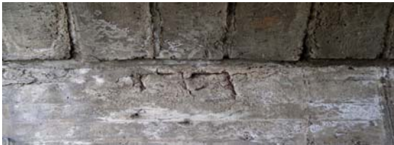
Figure 5: Damage of pier cap beam
