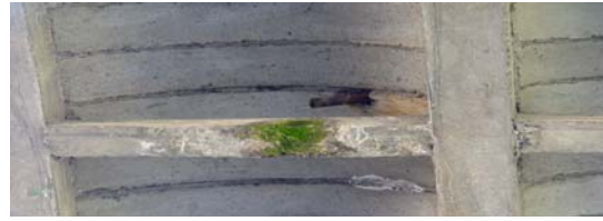
Figure 4: Damage of horizontal tie beam
