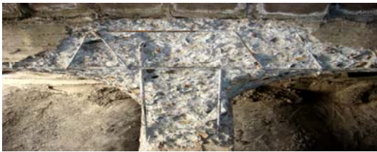
Figure 7: Damage of pier and pier cap
