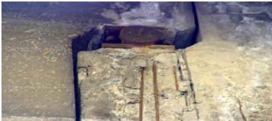
Figure 9: Damage of bearing and corbel
