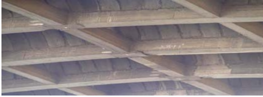
Figure 3: Damage of arch ring
