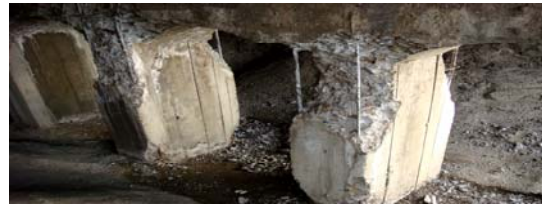
Figure 6: Damage of spandrel arch piers
