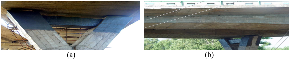
Fig. 4 Strengthening of the transverse beam of Y-shaped piers: (a) front view, (b) side view
