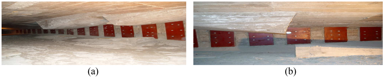
Fig. 3 Strengthening of box girders web: (a) right web of box girder, (b) left web of box girder
